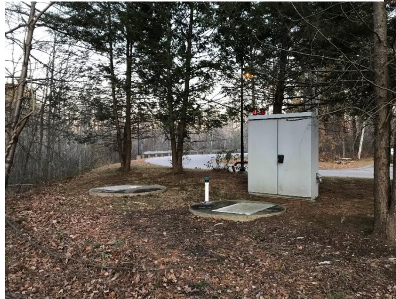
Photo: Seacoast Community School Pump Station
